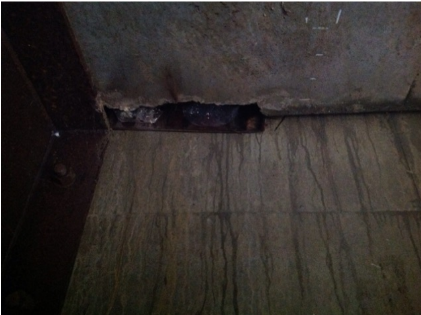
deck panel damage at left bank
