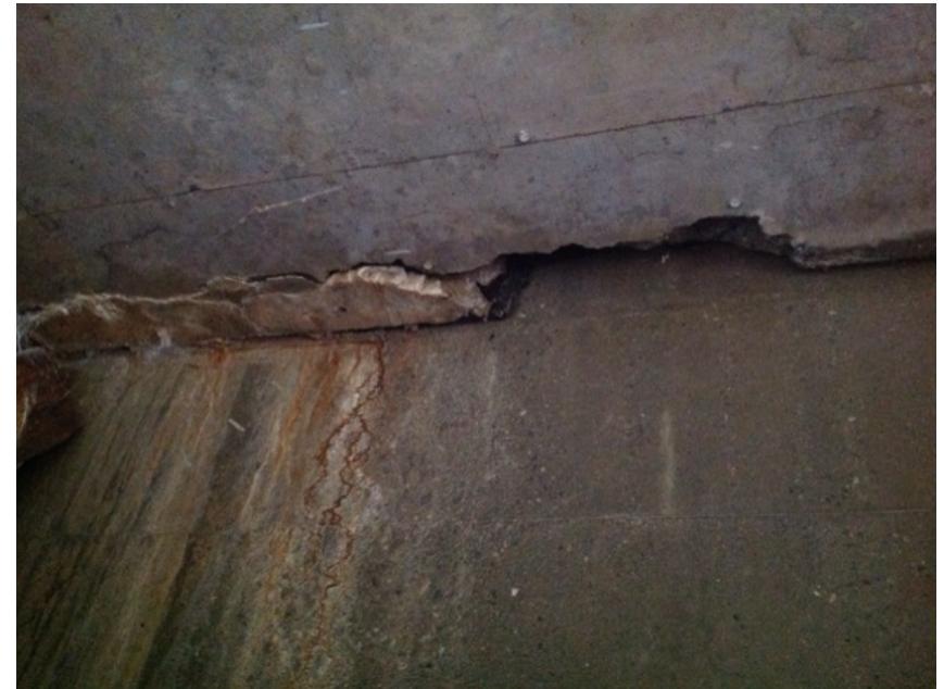
deck panel damage at right bank
