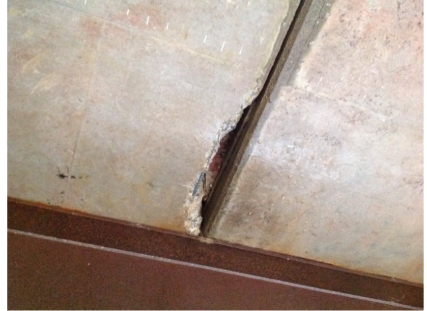
deck panel damage and rebar exposed
