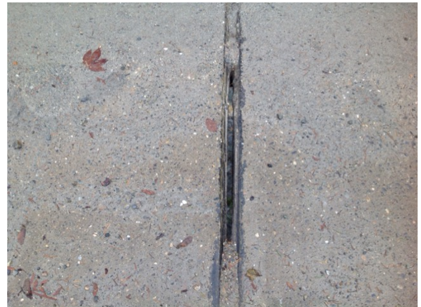
deck seals missing in some locations
